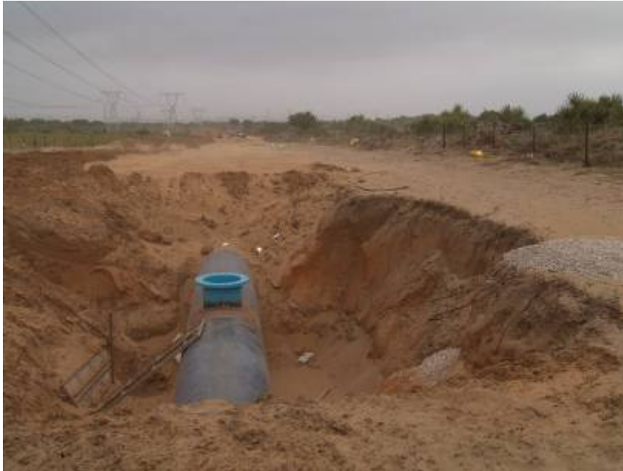
Figure 8: Construction of a pipeline in a servitude. Note the extensive clearing of vegetation
