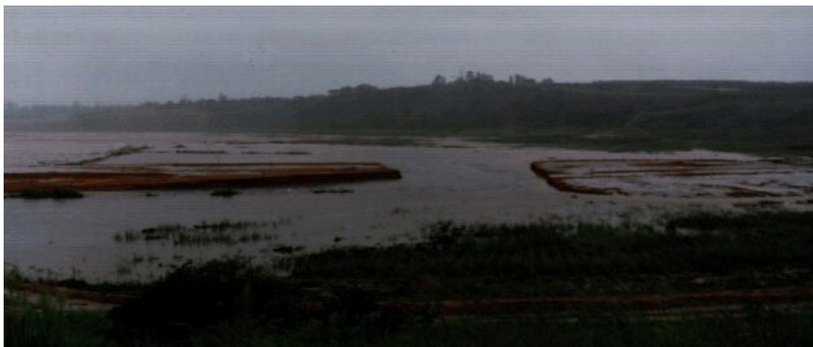
Figure 32: Flood damage to slimes dam (Photo: D Cyrus)
