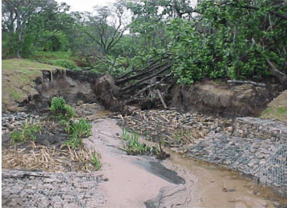
Figure 34: Damage to the stream channel in Alton due to undercutting of the stream bed (Photo: B Kelbe).
